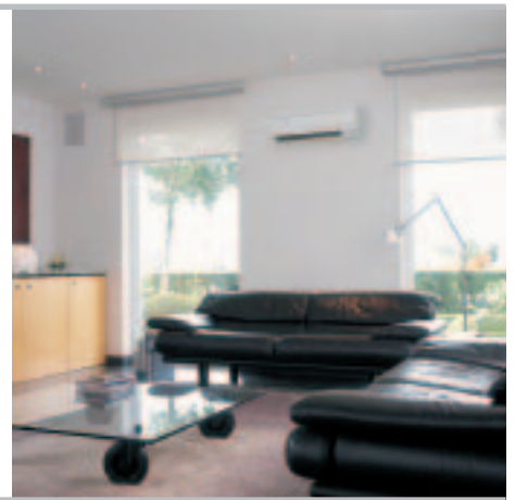
Wall mounted unit >
